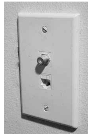
Figure 5-2: This wall plate combines TV and data network outlets.
